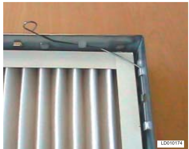
FIG. 34 – FULLY INSTALLED FILTER
