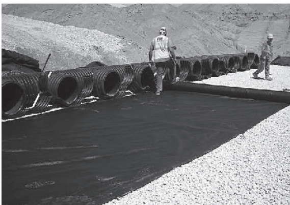
Install manifolds and lay out woven scour geotextile at inlet rows [min. 17.5 ft (5.33 m)] at each inlet end cap. Place a continuous piece (no seams) along entire length of Isolator® Row(s) in two layers.
