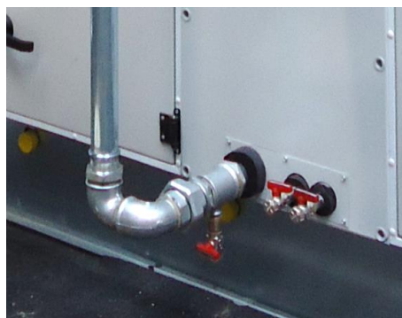
Figure 16 – Heat exchanger drains in installed condition
