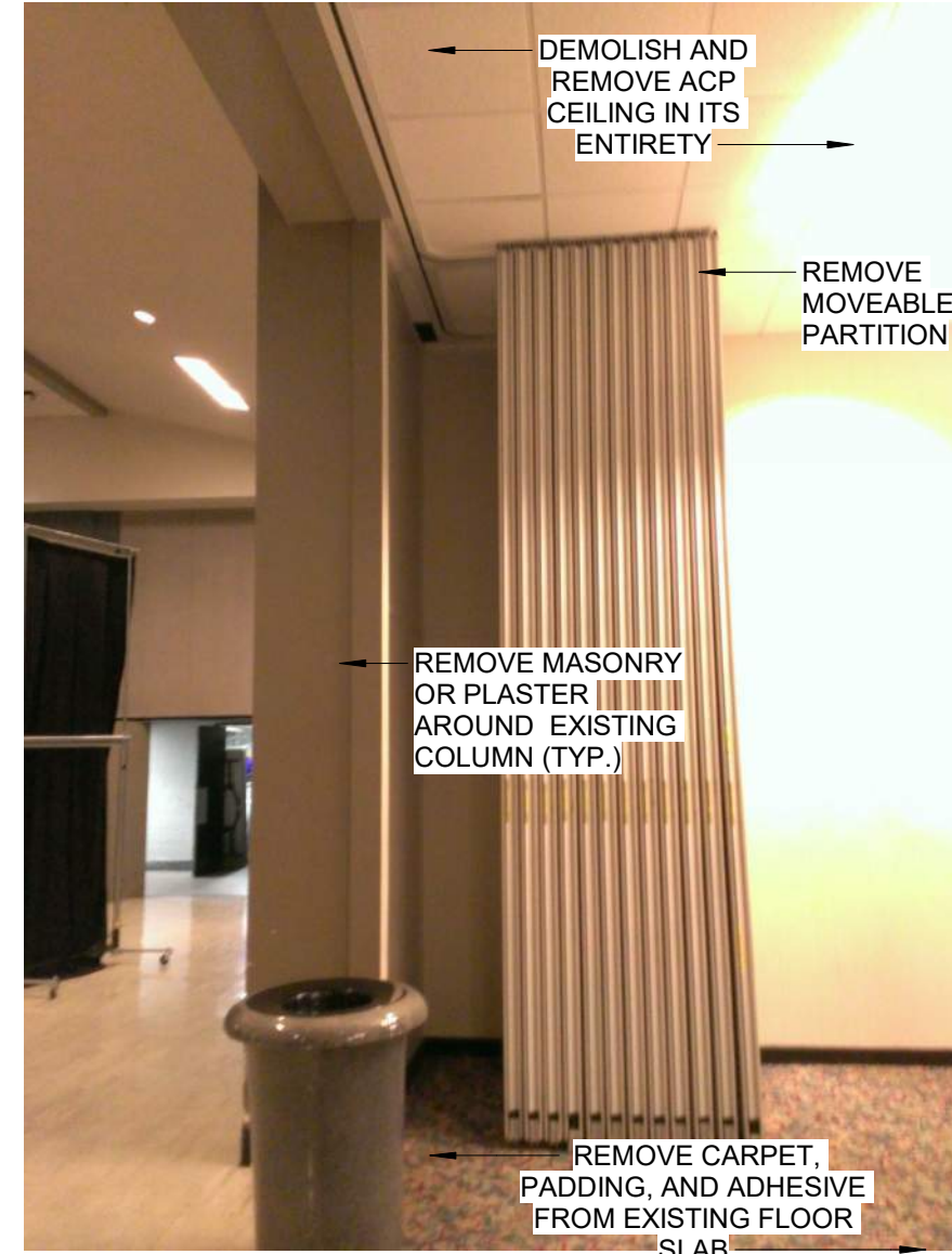
6 MOVEABLE PARTITION IN SMALL BALLROOM SD4.21
