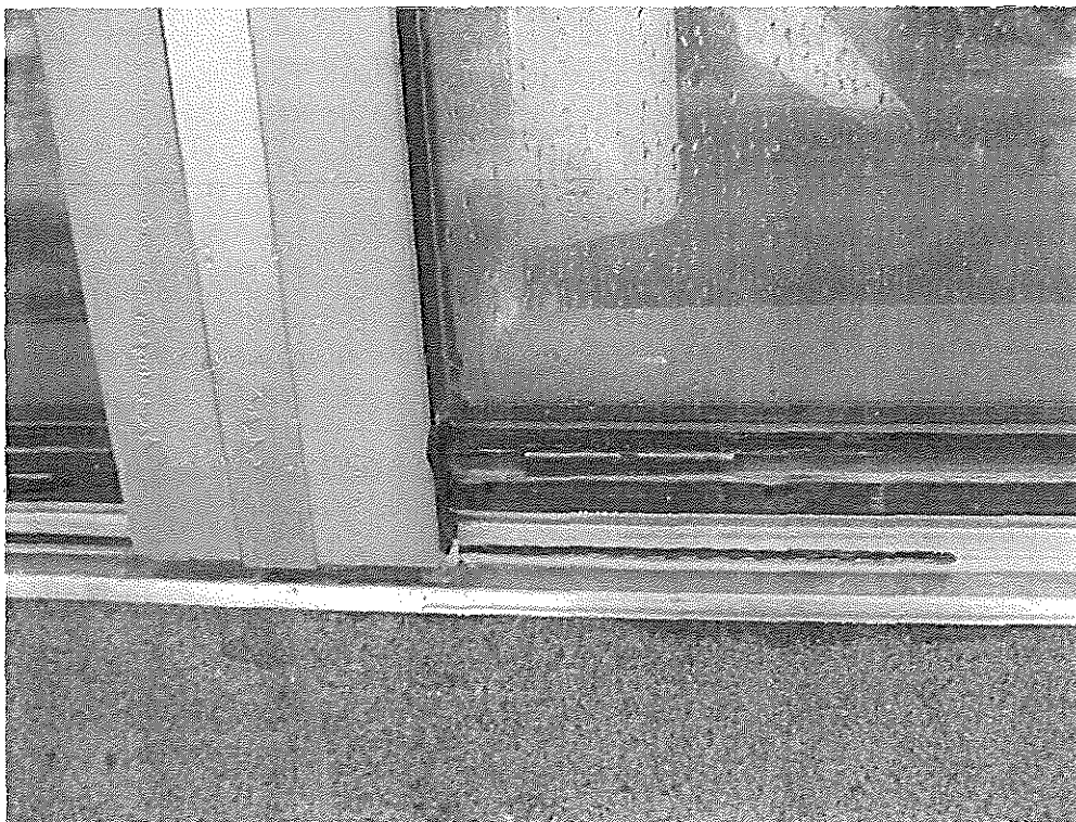
Photo No. 6: Exterior view of Specimen #3 at leak area with pressure plate and sealant joint removed
