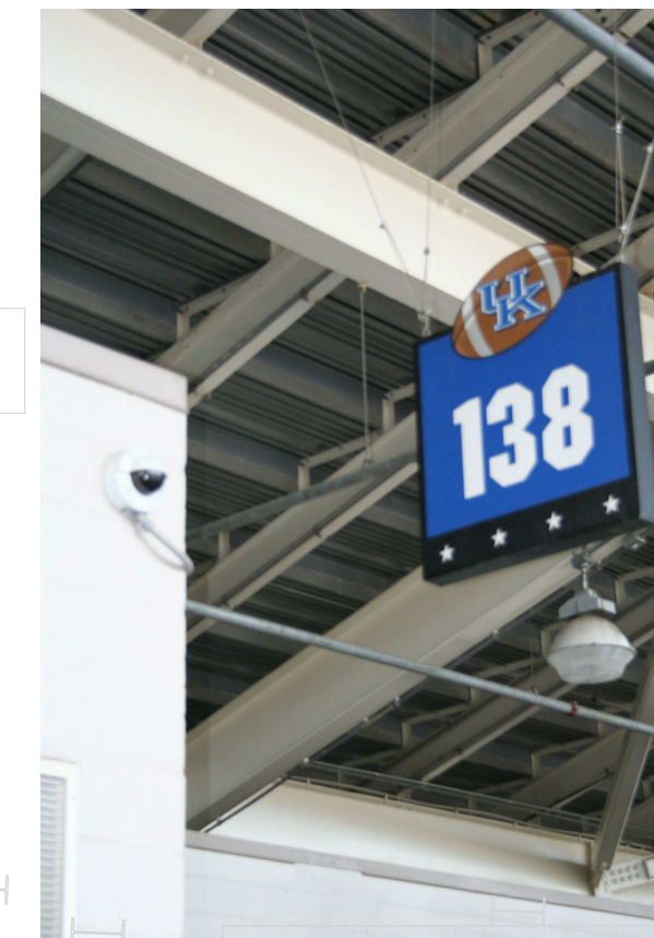
EXISTING CAMERA (EX.#16)
